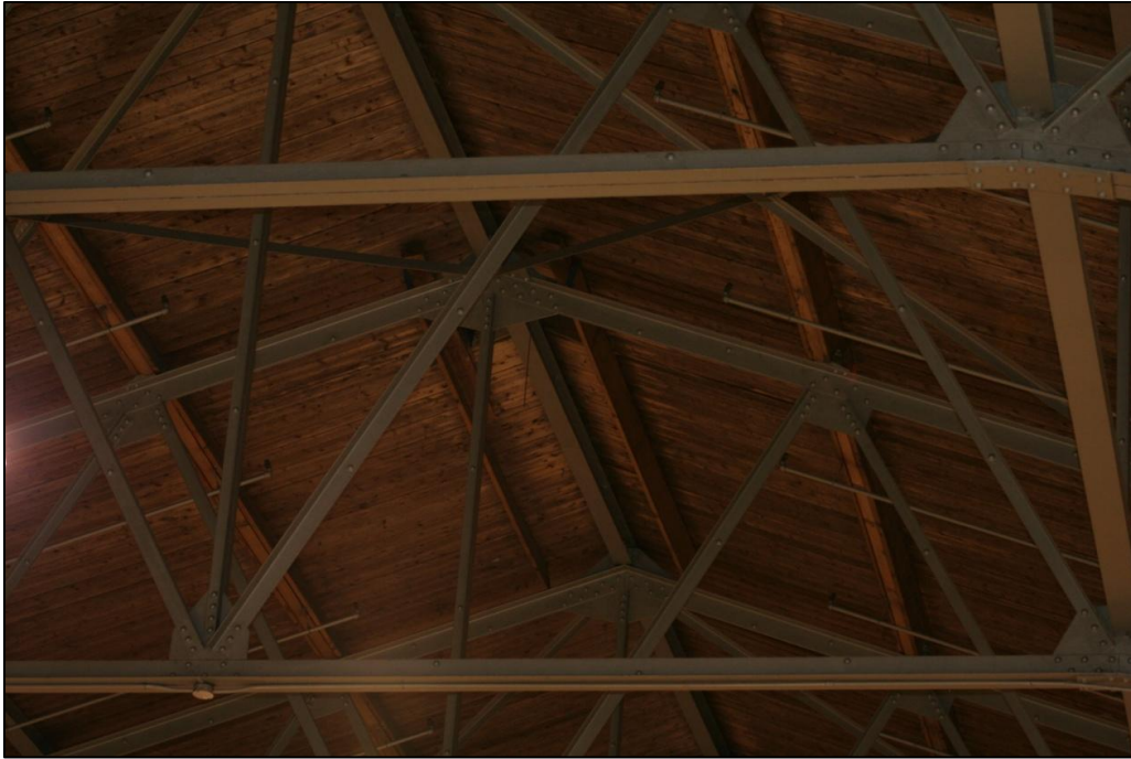
Plate 36: The truss work, wood supports, and wood used for the roof as visible in the Memorial Arena interior.
