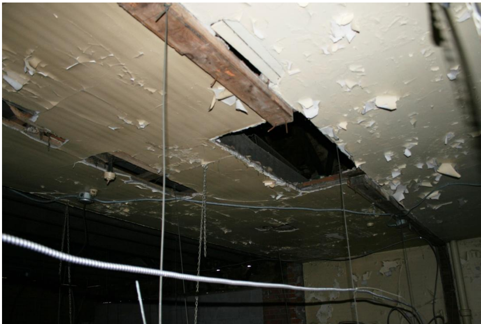
Plate 55: Above the false ceiling in the Weigh Scale Building. Note the use of lath-and-plaster.
