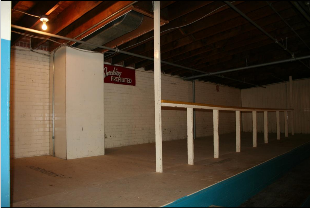
Plate 40: The standing room area in the Memorial Arena. Note the signage.
