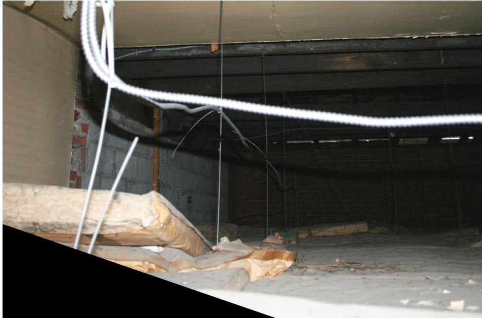
Plate 54: Above the false ceiling in the Weigh Scale Building. Note the beam structure and where the wall and roof coverings end.
