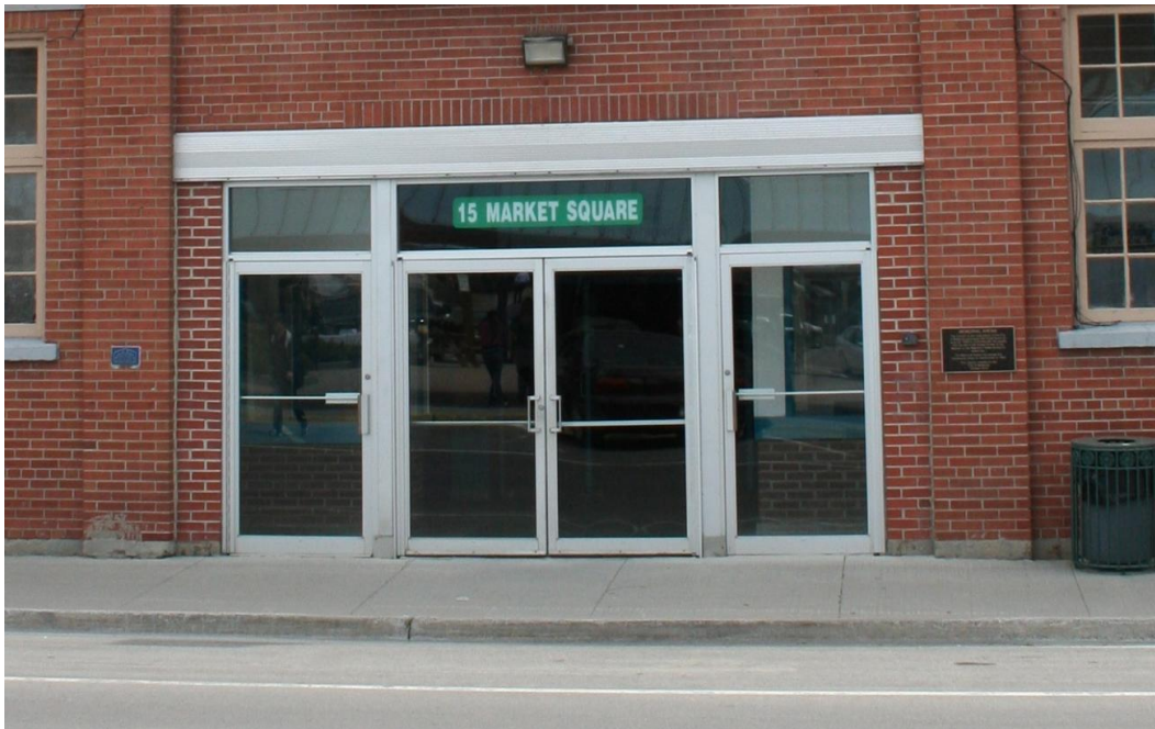
Plate 30: Entrance for the Memorial Arena. Note the different coloured bricks around the door, and the original size of the entrance.
