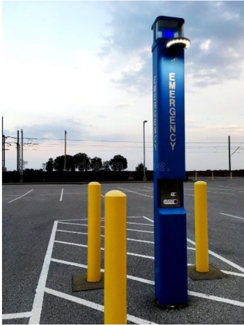
Emergency call station
