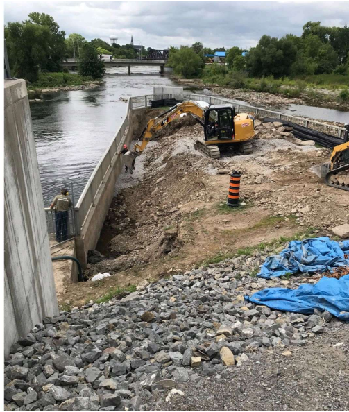
The beginning of placement of the pea stone and drainage tile. Picture taken looking downstream.
